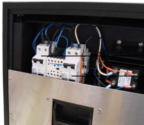
Main Circuit Breaker
